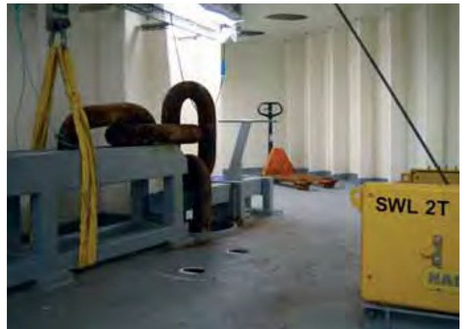
Electric Wire Rope Winch Type 42/87 E capacity: 2 t used for service work on the platform's anchorage chains
